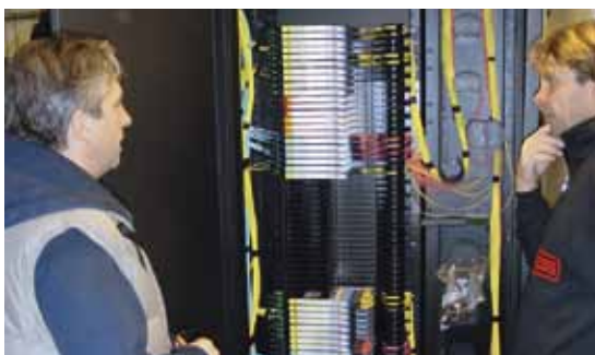
Sören Westerberg, 3 Sweden, and Hempa Jääskeläinen from installer Installateur Node Access, setting up the LiSA system.
